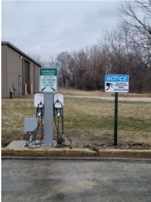
The car charging station located on the northwest end of the student parking lot on the Main Campus in South Holland, Illinois.
